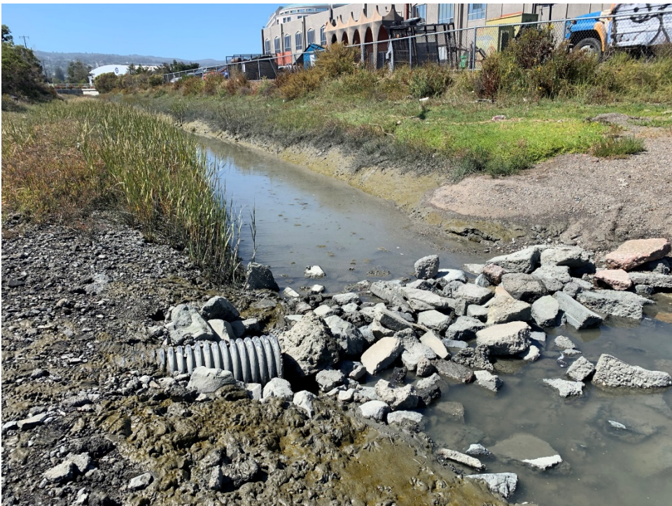
Photo 4. Existing stormwater outfall (to be replaced) near the mouth of Easton Creek, looking west at low tide.
